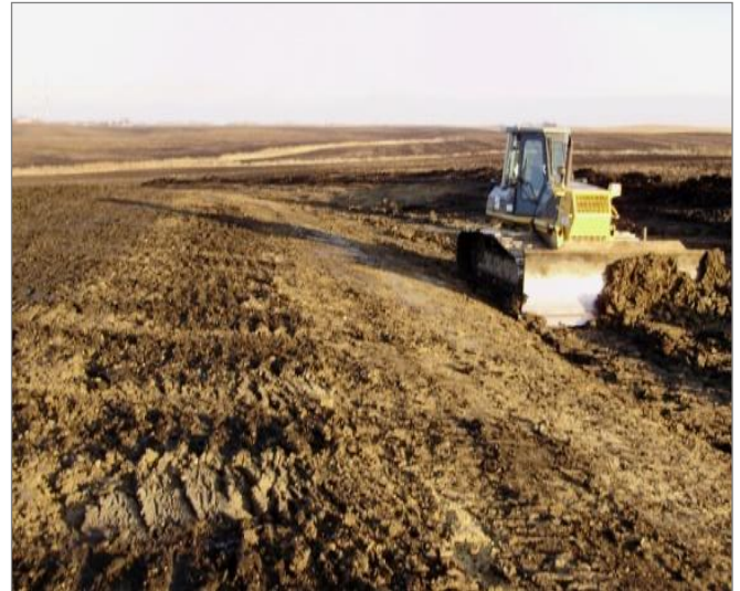
Gully being closed after tile and sediment basin installation as part of the Hay Creek Watershed Project.
